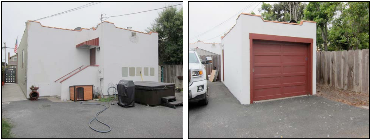
Figures 4 and 5. Left image shows the rear elevation with replaced stucco wall cladding. The rear yard between the house and garage was paved circa-1985 when the house was converted to law offices. Right image shows the garage's west elevation, taken from the 16 th Street alley.
