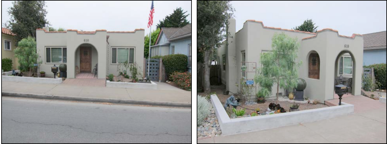
Figures 2 and 3. Left image shows the front elevation with central front porch and replaced front entry door, replaced vinyl windows and replaced stucco exterior wall cladding. Right image shows the front and left side elevations. The chimney has been encased in stucco and all windows have been replaced with vinyl-sash or vinyl-slider windows.
